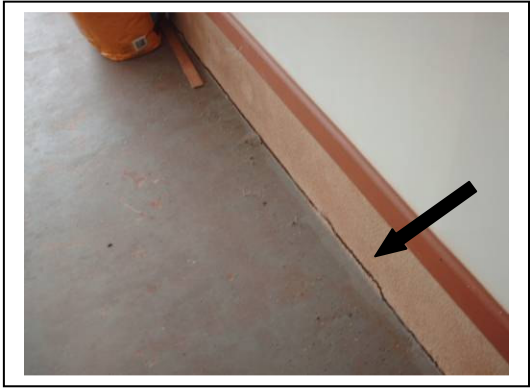
Garage floor settled somewhat
