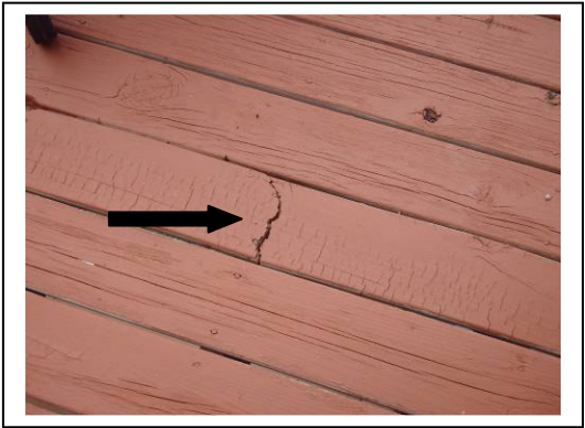
Damaged/broken walk board at the deck
