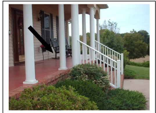
No porch rails at the front porch
