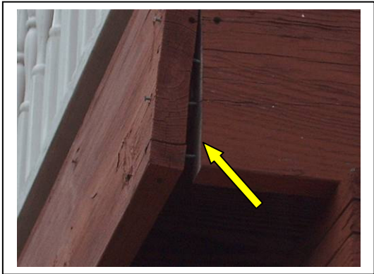
Loose boards a the deck
